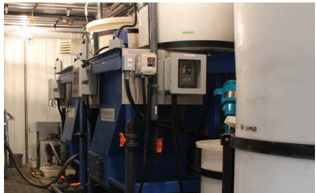
Lamellar clarifiers with instrumentation
