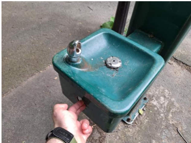
Figure 7.8: Broken water fountain Source: (Imbeau 2025)
